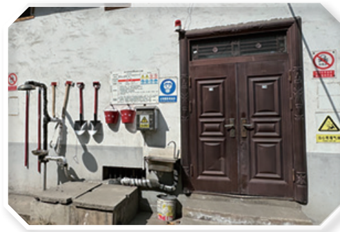
Safety equipment outside the chemical storage facility 化學物品庫外的安全設備
