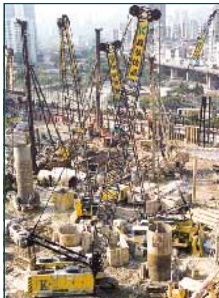
Bored piling and H-piling work at KIL 11127, Tai Kok Tsui, Kowloon, Phase 2 undertaken by KinWing Foundations Limited
