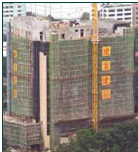
Superstructure work for Fanling Magistracy Building at 1A, Pik Fung Road, Fanling, New Territories undertaken by Chinney Construction Company, Limited
