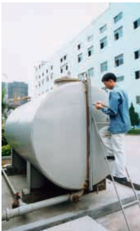
Regular checking on fuel storage for in-house power generator 定期測量廠內發電機之燃油儲備
