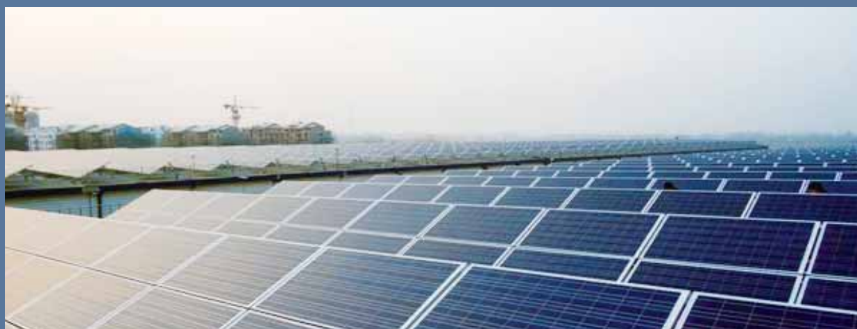
Suqian Rooftop Photovoltaic Energy Project 宿遷屋頂光伏發電項目
