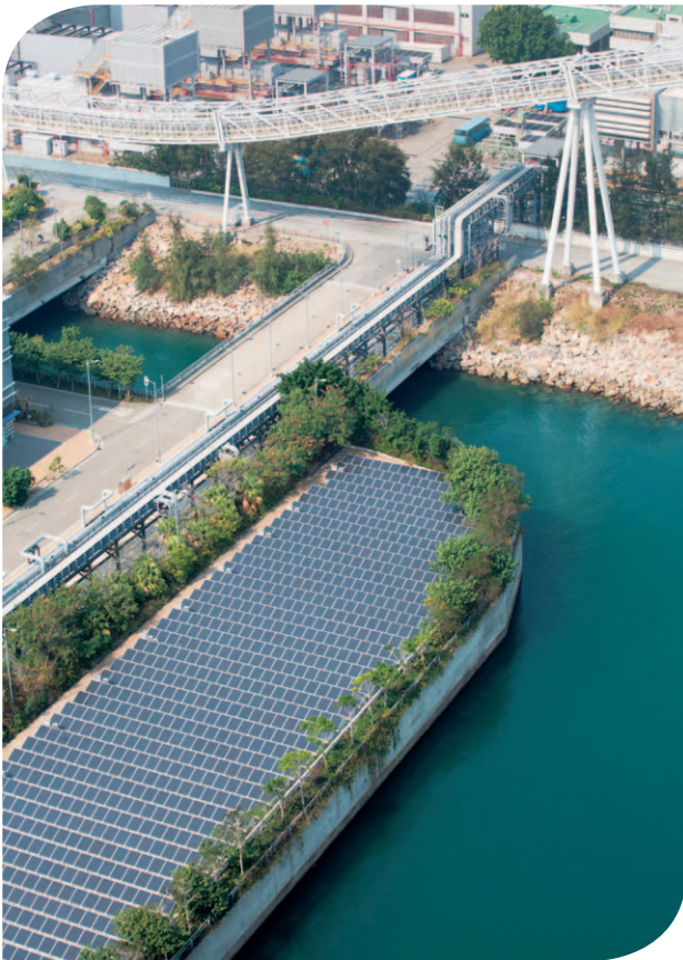
HK Electric's solar power system helps reduce carbon footprint.
