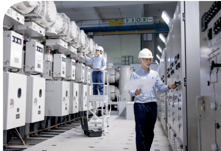
North Point Switching Station is upgraded with new compact switchgear.
