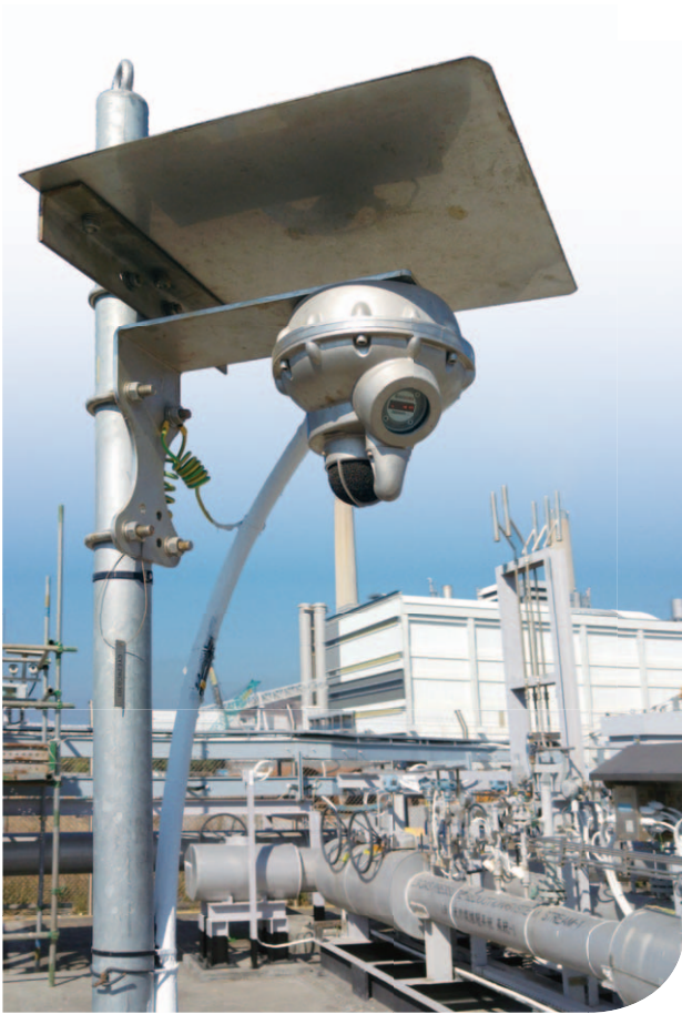
Acoustic sensors installed to enhance the safety infrastructure of Lamma Power Station.
