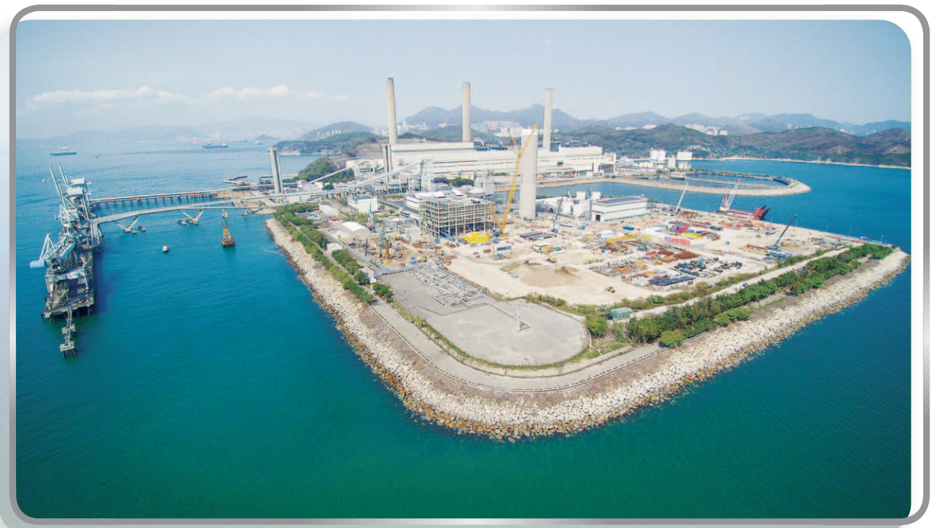
Lamma Power Station is undergoing major construction works to increase its gas-firing generation capacity.
