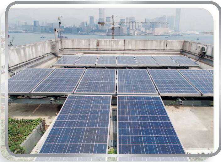
Solar panels on substations help reduce our own carbon footprint.
