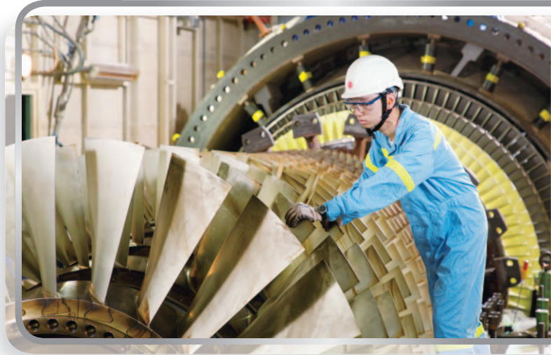
An engineer at work on the L9 generating unit to ensure its safety and performance.
