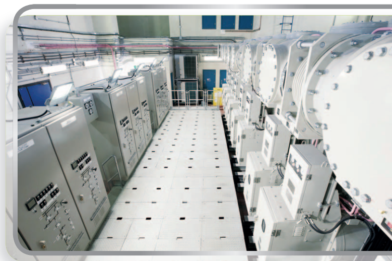
North Point Switching Station undergoes network security upgrades to maintain the reliability of the system.
