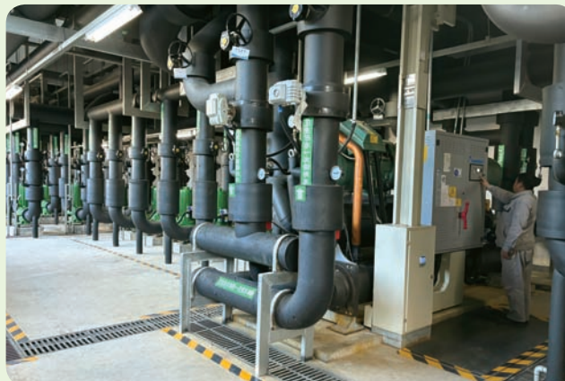
Daxing branch factory's ground source heat pump system 大興分廠地源熱泵系統
