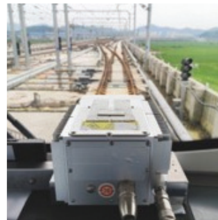
Installed on trains (interior view)
