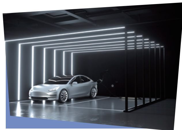
Charging station at Chengdu ICD Mall 成都環貿ICD充電場站
