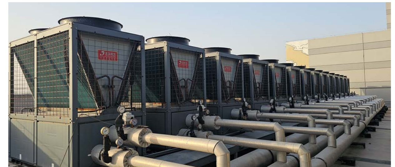
Peak Shaving and Energy Storage at Dongying Wuyue Plaza
