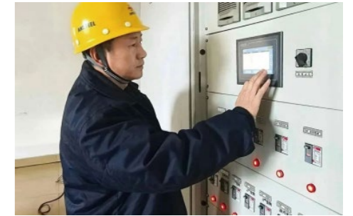
Heating System Monitoring
