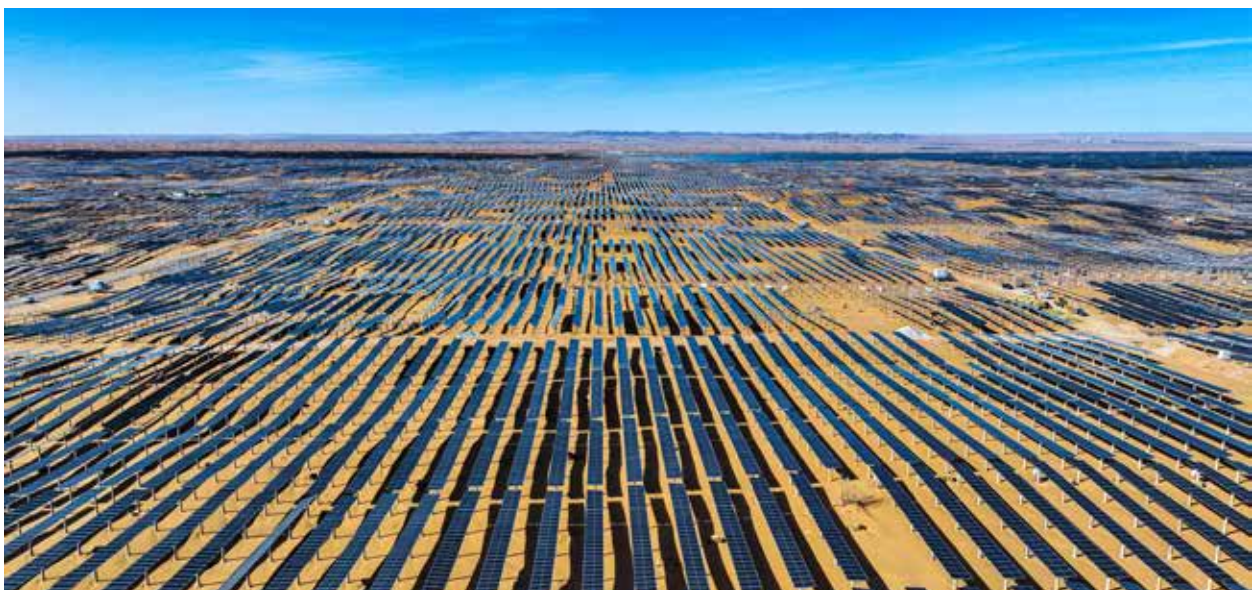
Ningxia Tengger "Shagehuang" new energy base
