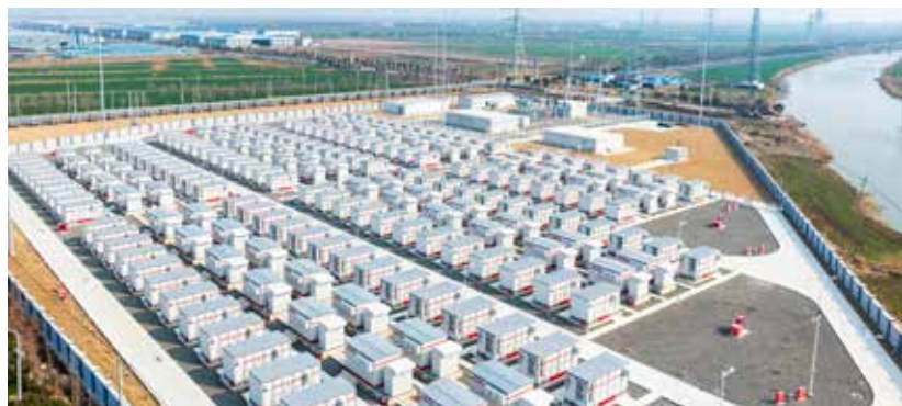
Longyuan Jiangsu Sheyang Shared Energy Storage Power Station
