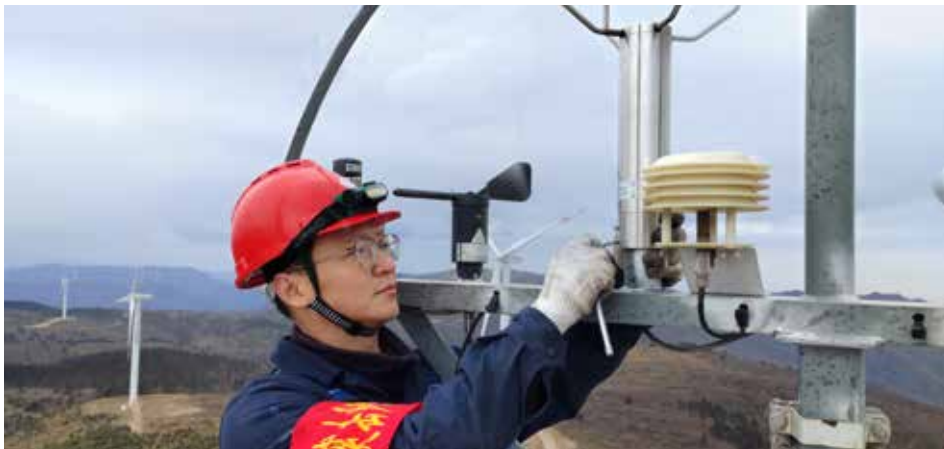
Installation of heated ultrasonic meteorological instruments
