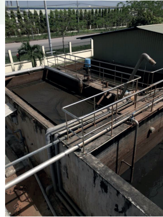
Wastewater treating facilities in Dream Textile
