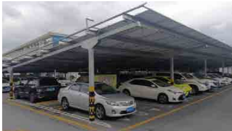
Photovoltaic Installation on Parking Lot Rooftops
