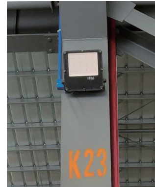
LED lighting in production workshop
