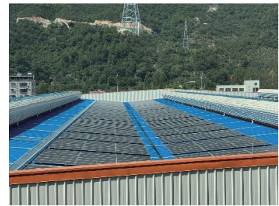
Solar Photovoltaic System
