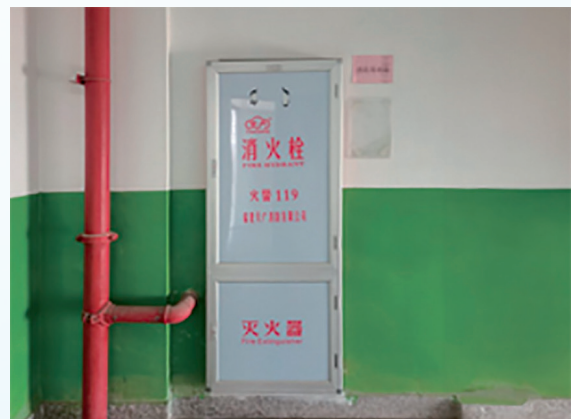
Fire Fighting Equipment
