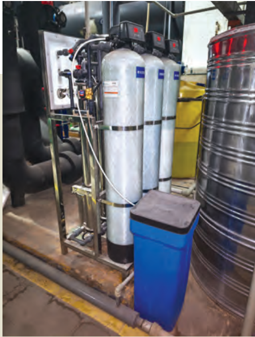
Reverse osmosis filtration systems are installed in COP to reduce water usage in pools and fountains
