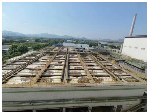
Wastewater treatment facilities within plants
