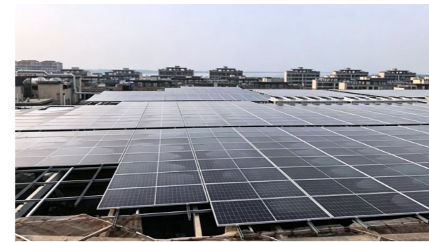
Rooftop Photovoltaic Installation at Suzhou Xinghu Paradise Walk
