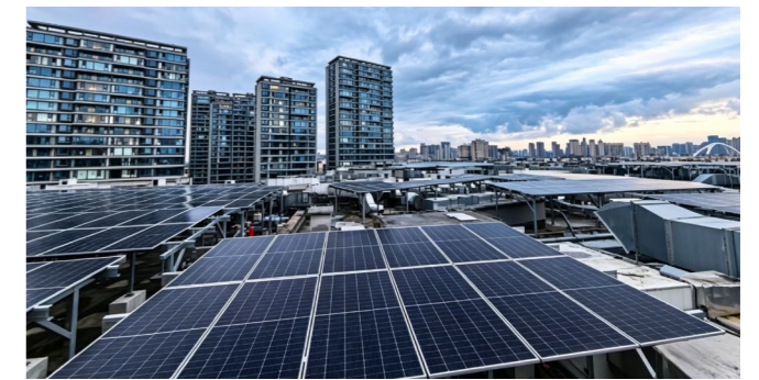
Rooftop Photovoltaic Installation at Ningbo Haishu Paradise Walk
