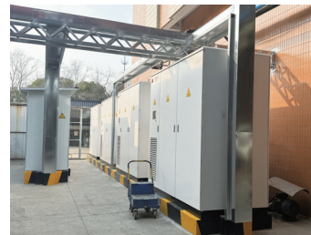
Energy Storage Project
