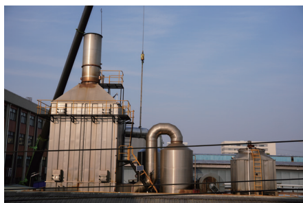
Waste gas treatment device at the sewage station of Yadong (Changzhou) before renovation
