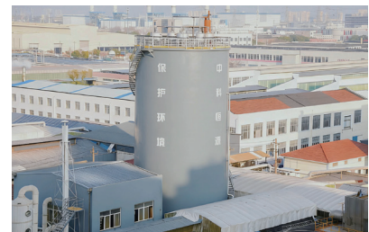
Anaerobic Tower at the Sewage Treatment Station of Yadong (Changzhou)
