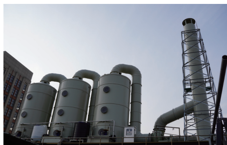
Waste gas treatment device at the sewage station of Yadong (Changzhou) after renovation
