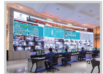
Jinma Energy Production Control Center
