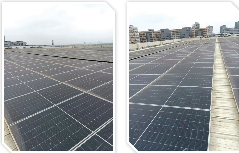
Roof-Mounted Photovoltaic Power Generation
