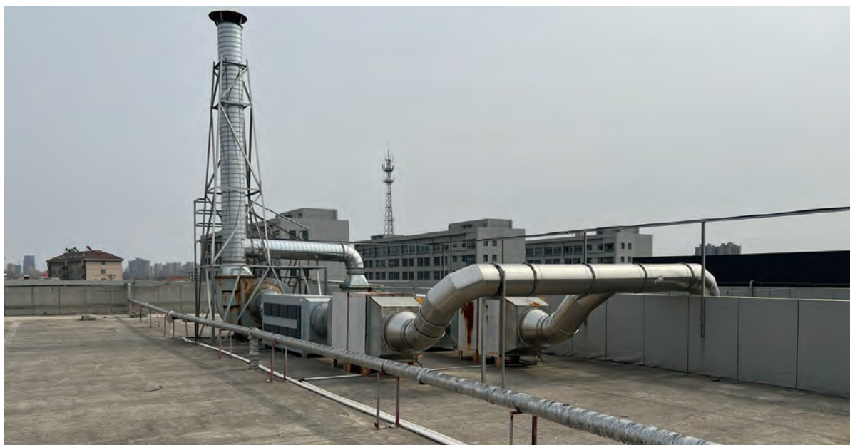
Activated carbon and photo-oxygen catalytic treatment equipment
