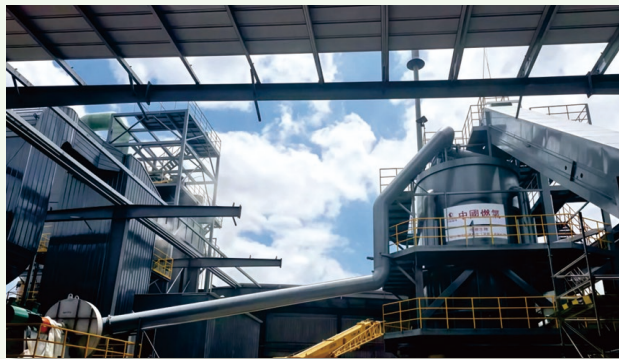
Nanjing Gotion New Energy Biomass Clean Heating Project
