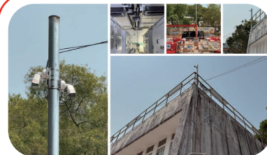
Smart Monitoring at Pui O Raw Water Pumping Station
